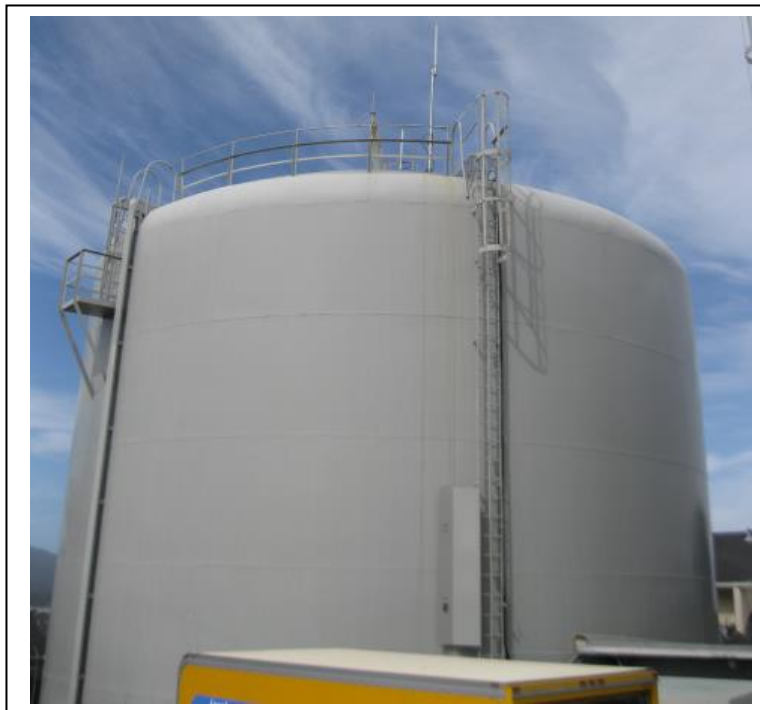
500KG Steel On-Grade South Tank
