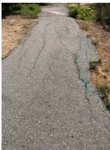
Asphalt Trail in Poor Condition
