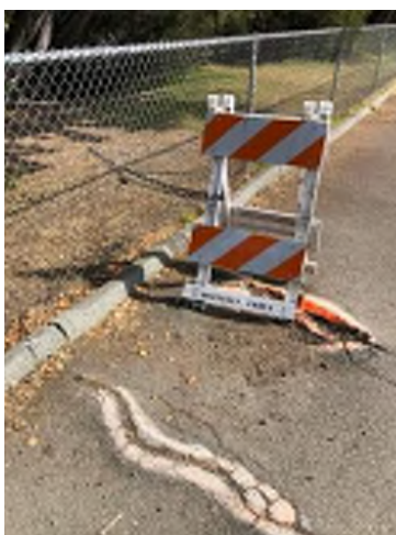
Asphalt Trail Root Impacts
