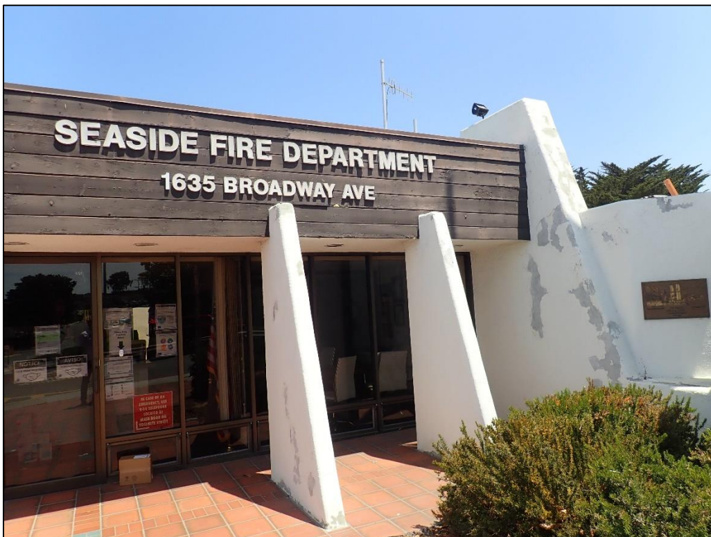
Brown paint on façade
