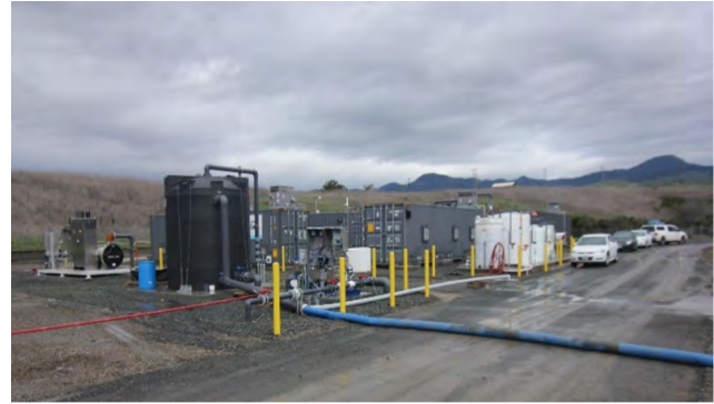
Cambria CSD Water Desalination Plant
