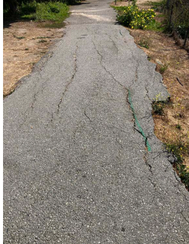
Asphalt Trail in Poor Condition
