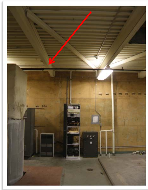
View looking northerly -arrow points to penetration
