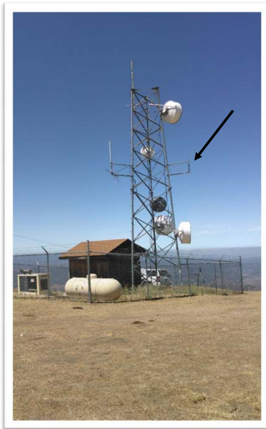
View looking westerly *Arrow points to vhf mount needing removal
