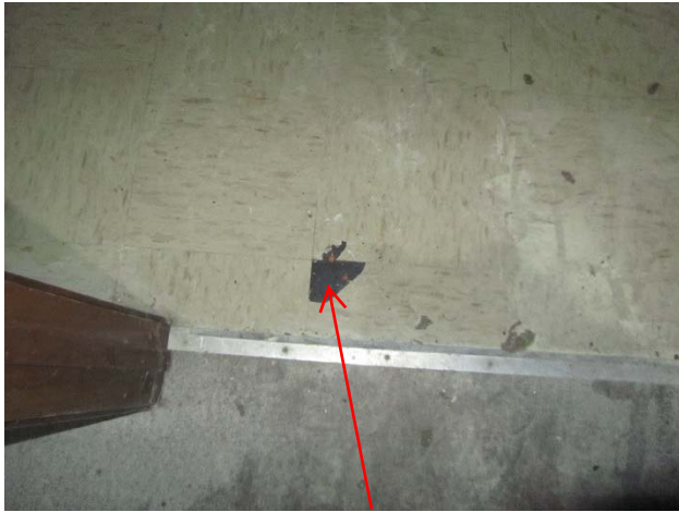
S - Asbestos Black Floor Tile & Mastic (2 nd Layer)
