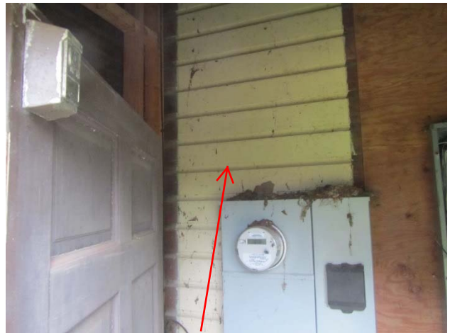
Lead-Based Paint on Wood Siding
