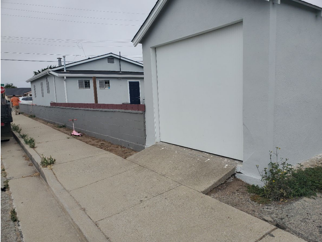
Existing, non-conforming driveway approach on Alhambra.
