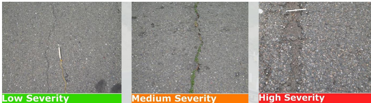
Image 4: Longitudinal and Transverse Cracking
