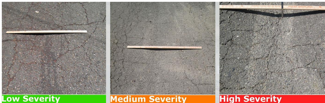
Image 6: Rutting and Depressions
