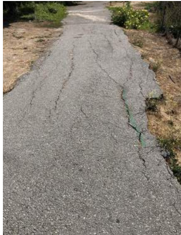
Asphalt Trail in Poor Condition
