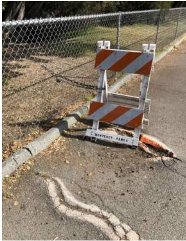
Asphalt Trail Root Impacts
