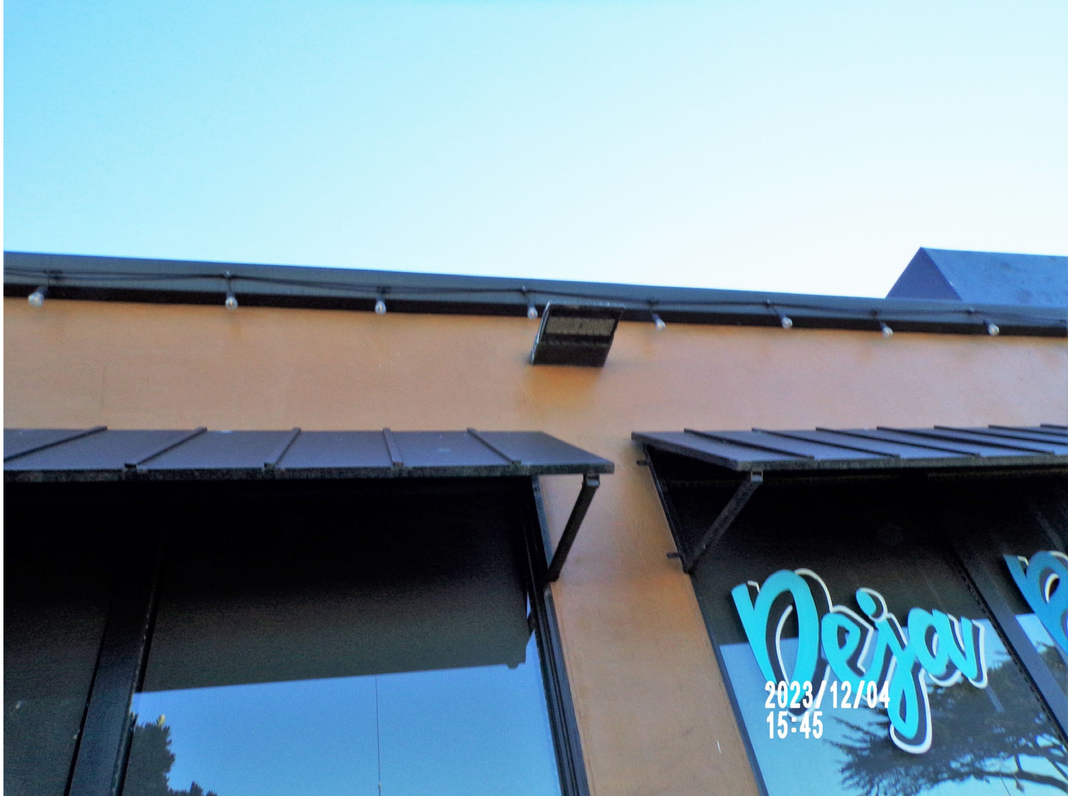
Picture 6: View of existing lights on 500 Broadway Ave.
