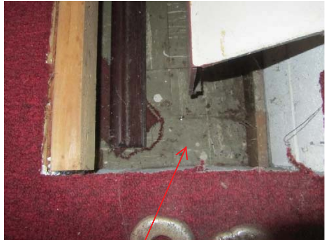
D - Asbestos Floor Tile & Mastic (under Altar)
