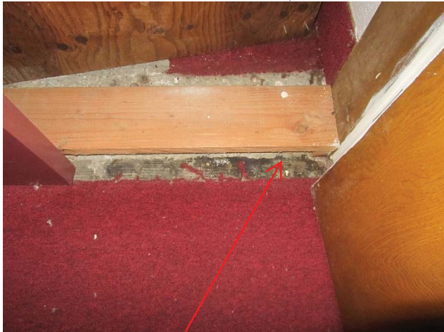
E - Asbestos Black Mastic (Under Carpeting)
