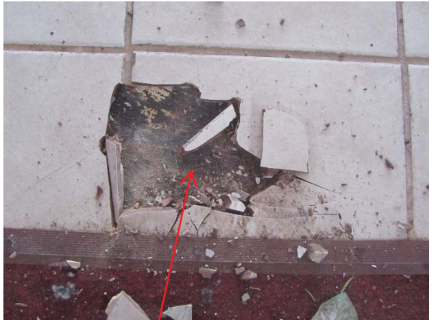
E - Asbestos Black Mastic (Under Ceramic)
