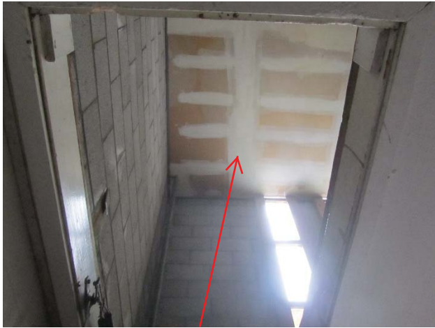
A - Asbestos Wallboard/Joint Compound
