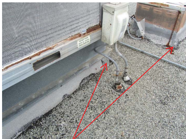
AA - Asbestos Roof Mastic
