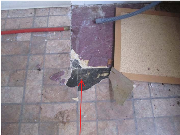
I & Z - Asbestos Black Mastic (Kitchen)
