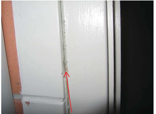
CC - Asbestos White Interior Door Frame Sealant
