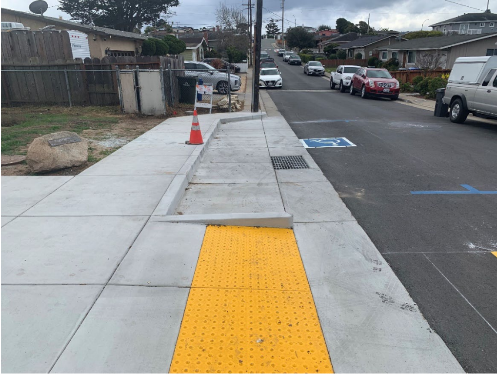
Example of recessed ADA compliant parking space being constructed on Lincoln St.
