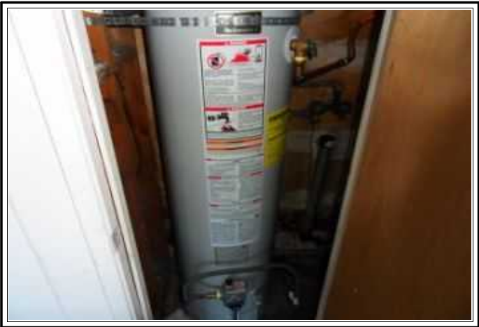
double-strapped water heater
