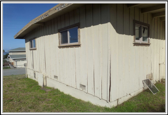
weathered wood siding
