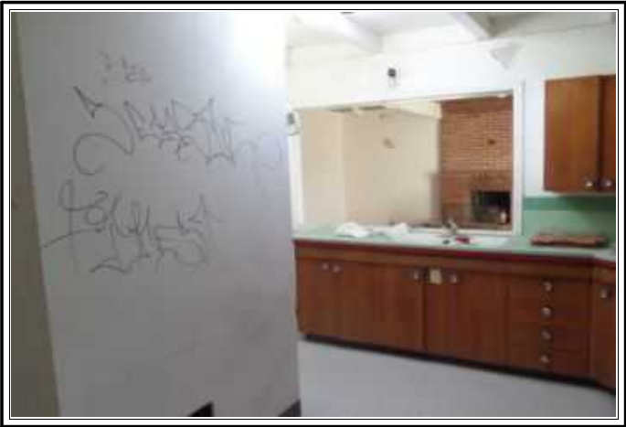
vandalism in kitchen
