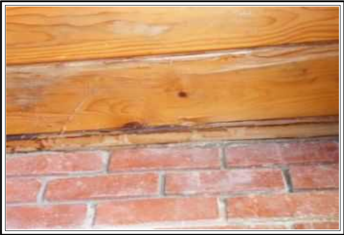
terminate damage on family room ceiling
