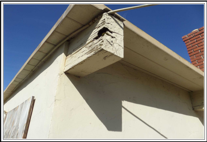
terminate and water damage
