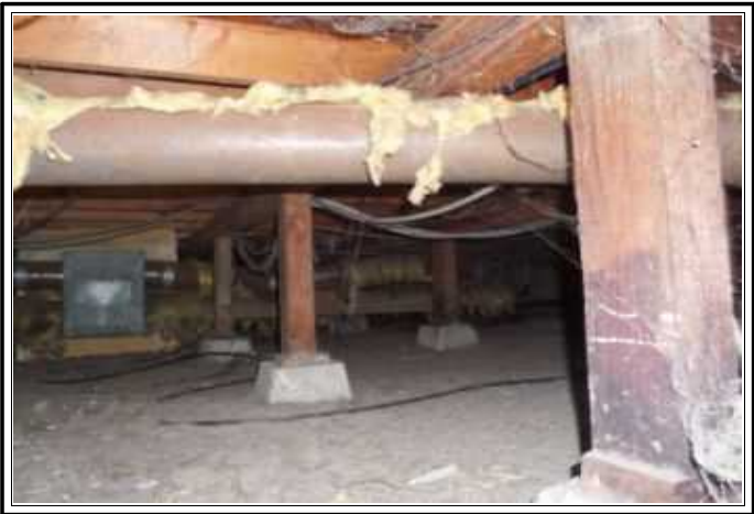
furnace and duct system underneath property
