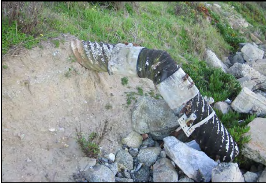
Figure 1-5. 12-inch corrugated steel drainage pipe
