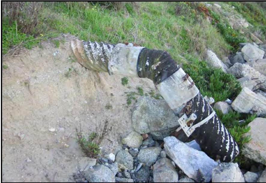
Figure 1-5. 12-inch corrugated steel drainage pipe
