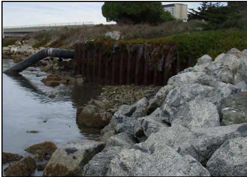
Figure 1-6. 20-inch oil delivery pipeline at the south end of project reach (view looking north).
