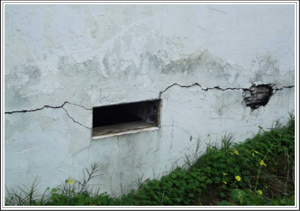
Cracking in stucco near foundation
