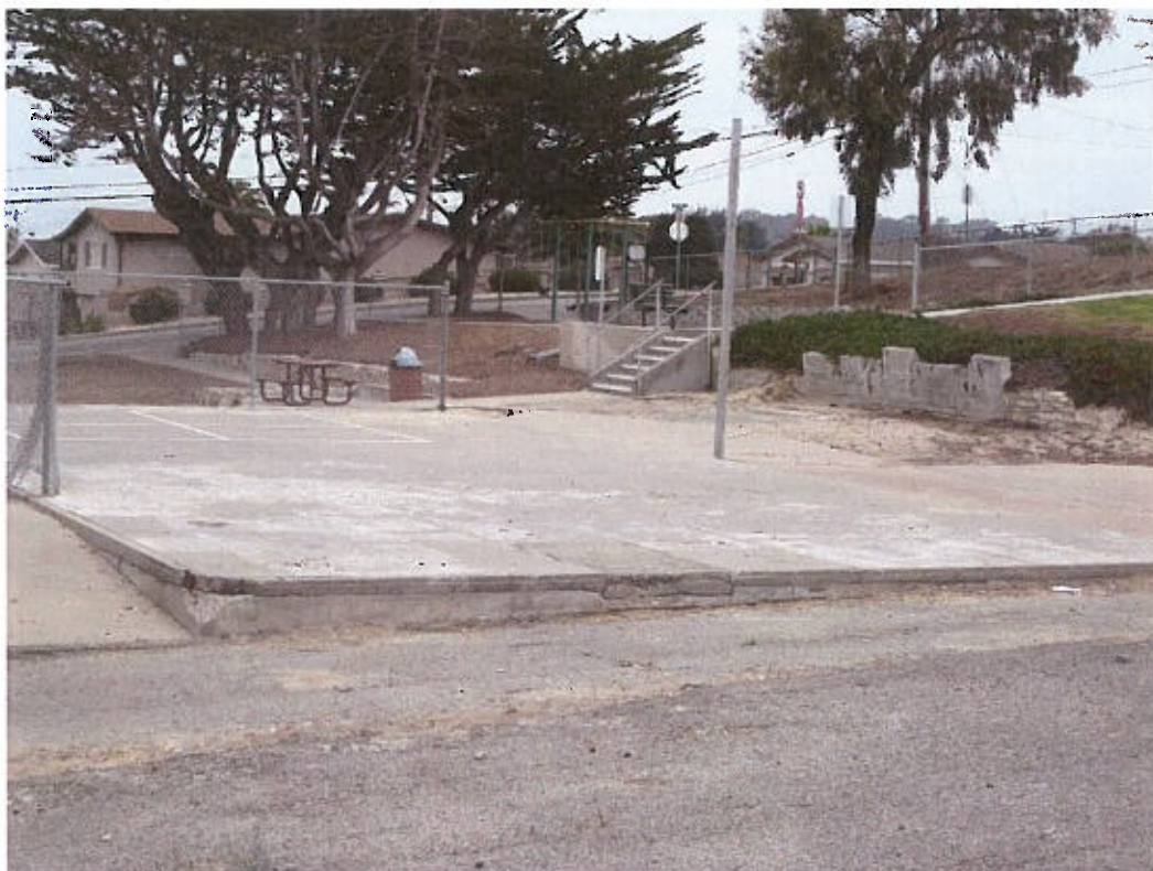
Capra Park basketball Court that needs rehab
