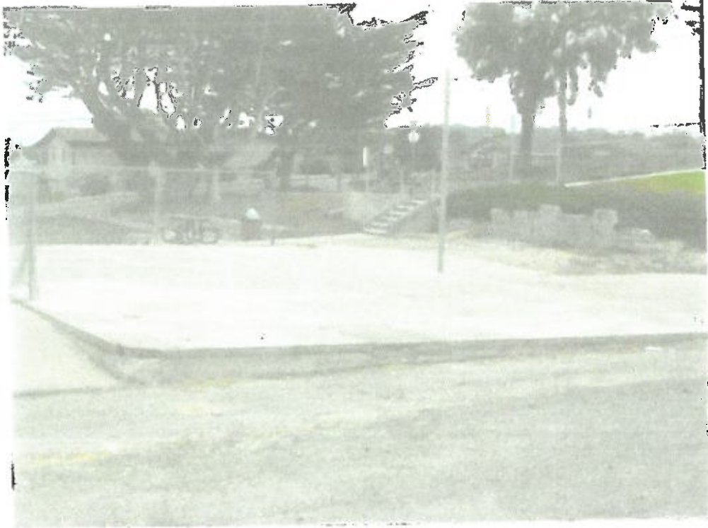
Capra Park basketball Court that needs rehab
