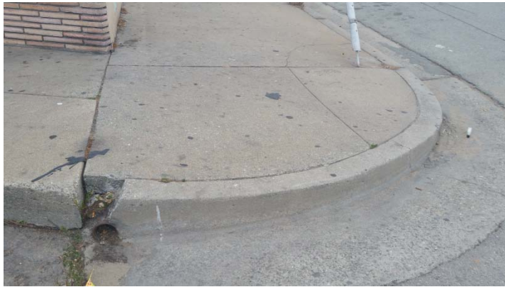
Figure 4. Existing non-ADA compliant curb, picture taken from corner of LaSalle and Frontage Road facing East
