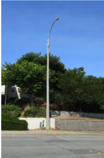
Light pole on intersection of Yosemite St. & Wanda Ave.
