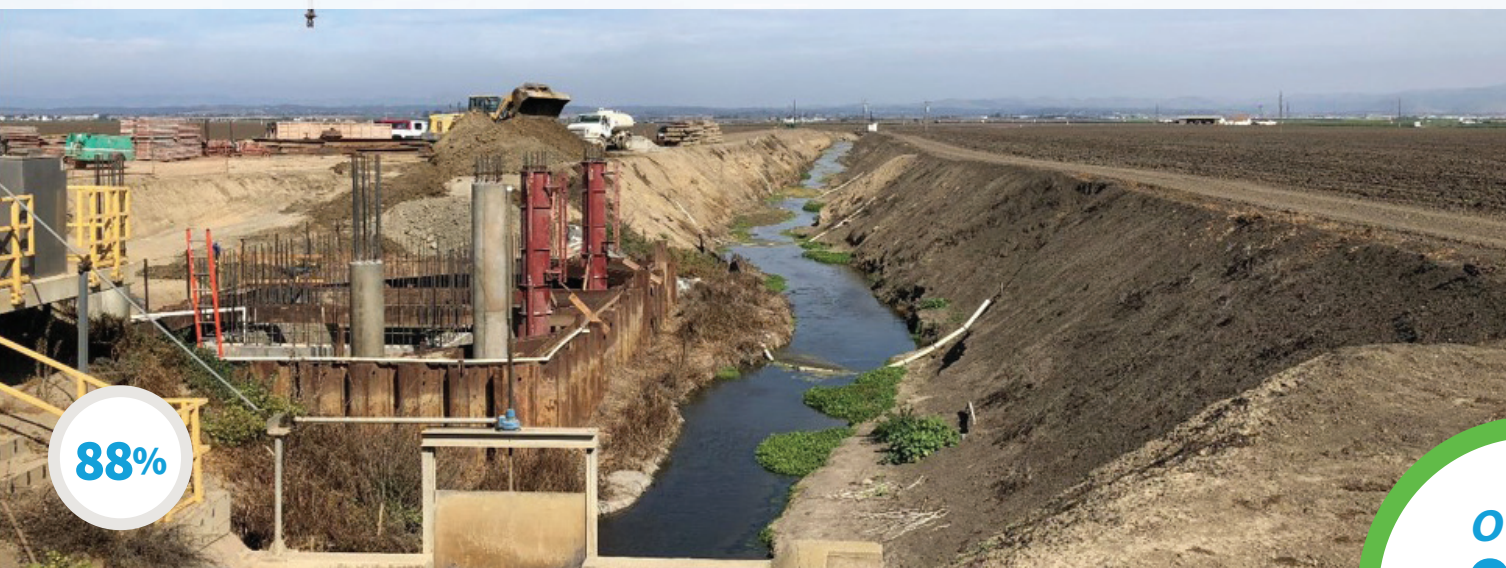
Source Water Diversion Structures
