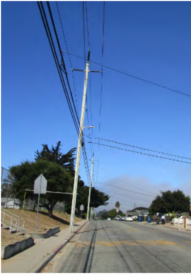
5th pole on Kimball Ave.
