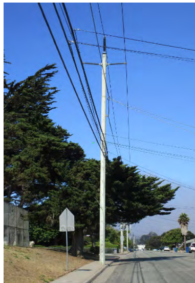
6th pole on Kimball Ave.
