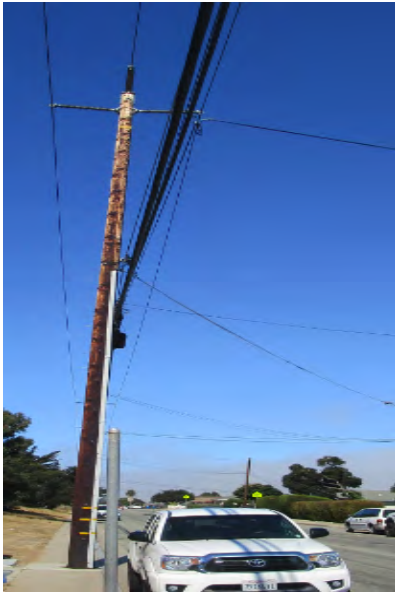
2nd pole on Kimball Ave.
