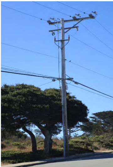
1st pole on Noche Buena St.
