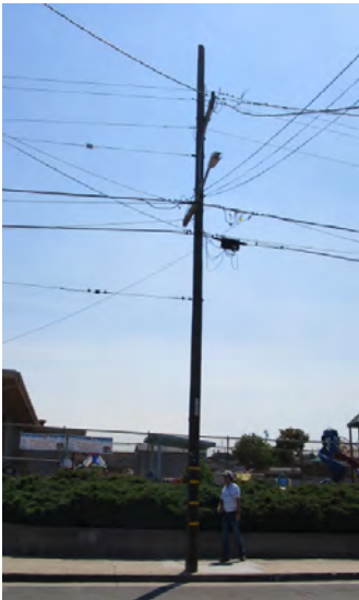
Pole is on Waring St.
