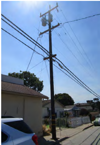
Pole is on Waring St.
