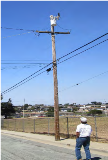
Pole is on Tweed St.
