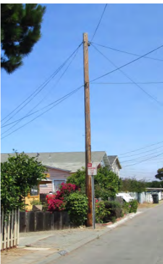
Pole is on Waring St.
