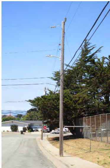
Pole is on Tweed St.
