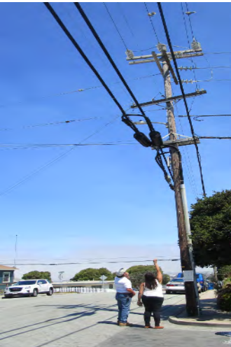
Pole is on intersection of Noche Buena St. & Wanda Ave
