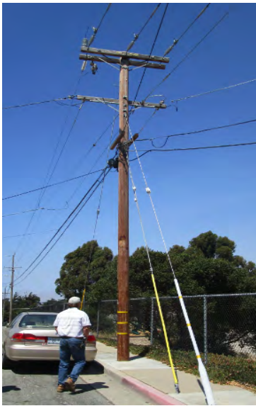
Pole is on Tweed St.
